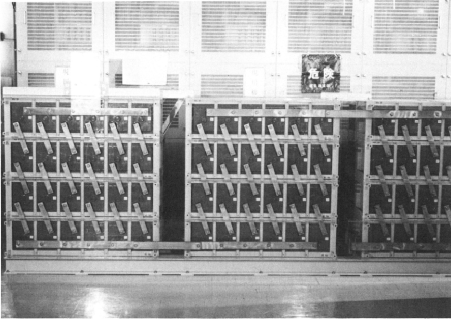
Fig. 16. Practical example of a unit of 23 batteries (3000 Ah).
